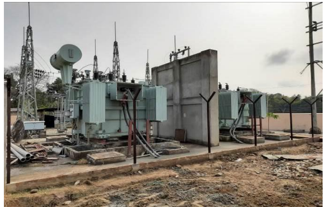
Fire Wall at 33/11 kV LGM Hospital S/S
