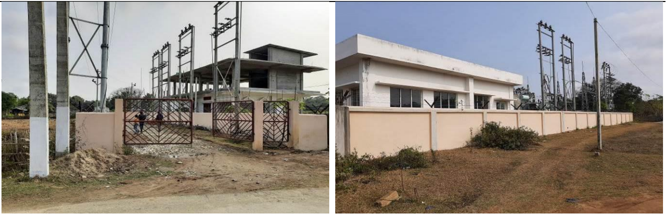
Boundary Wall and Gate at 33/11 kV LGM Hospital Substation
