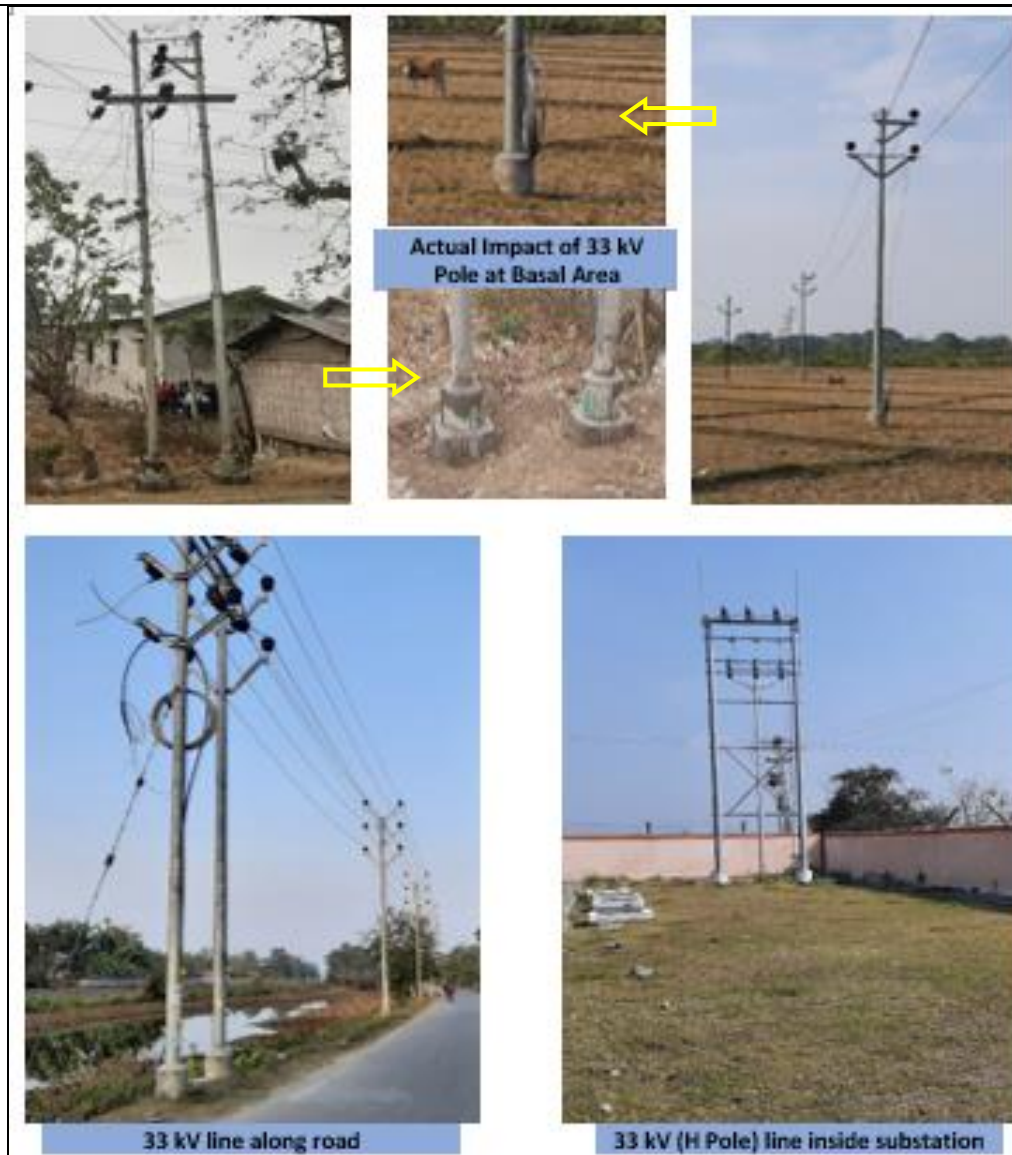
Figure 5.2: 33 kV Lines (Single & H Pole) Depicting Base Area Impact
