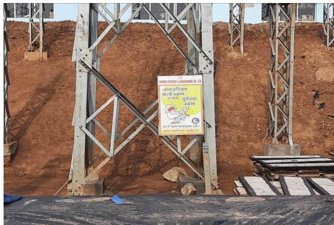
Condition of Limited Sign Boards
