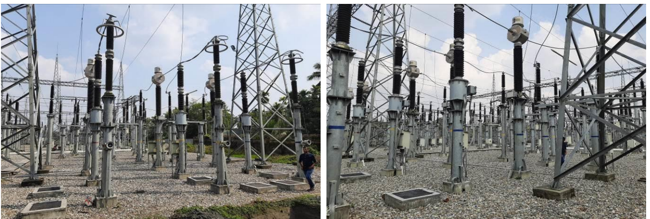
220/132 kV Rangia Substation (Bay Extension)
