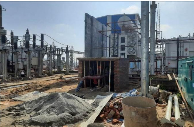
Fire Wall at 220/132 kV Amingaon GIS S/S
